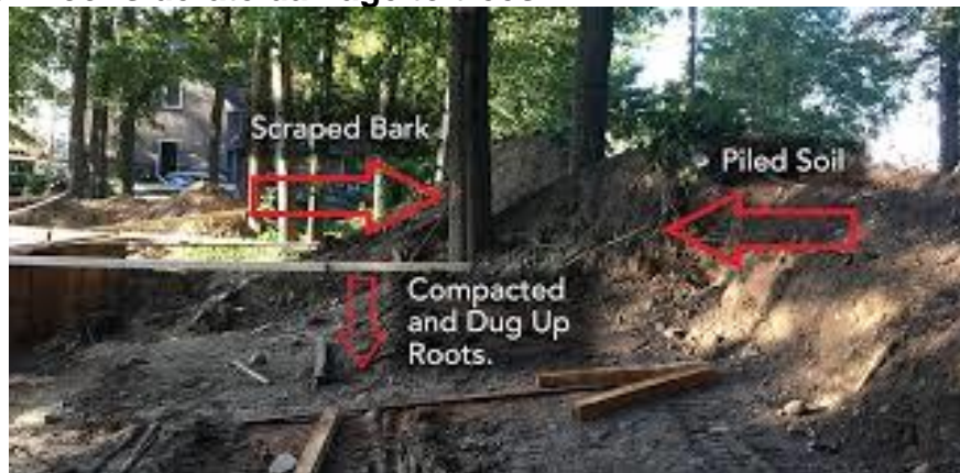
Image 6: Inconsiderate damage to trees
